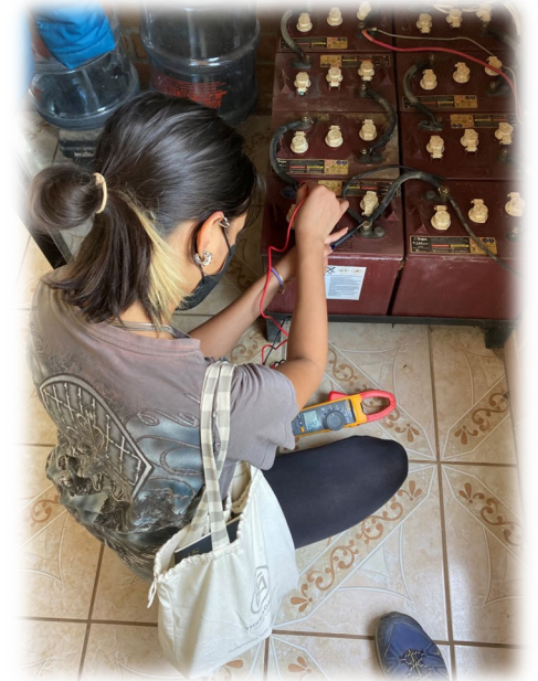
Joya measuring batteries at the Barbara Ford Center
